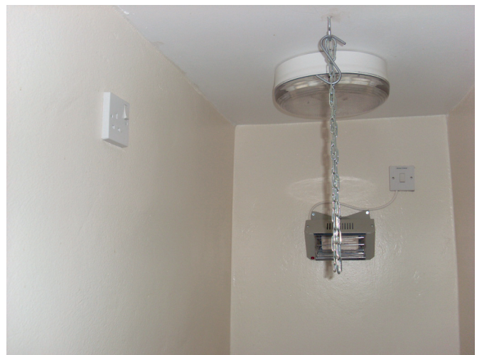
Fig. 34.3 Heat source, light and electrical points should be situated out of reach of the patient
